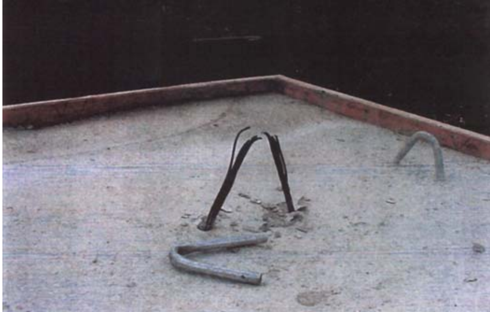
Photo 6. Pulling iron strand failure
